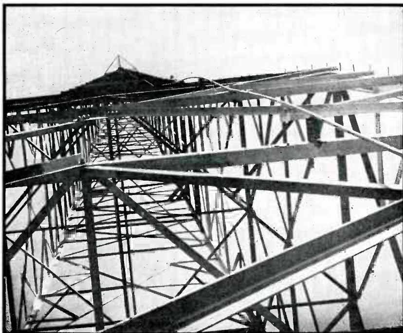
The concentric line feeding WBRL's square-loop f-m antenna at the top of WJBO's a-m tower is purposely left loose to allow for expansion and contraction. The line may be seen running up from the right
